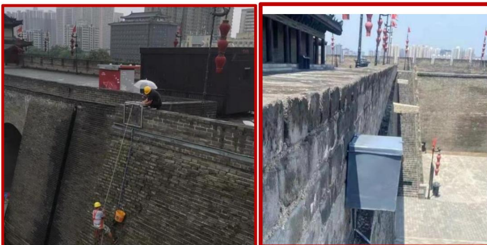
裂缝现场监测
